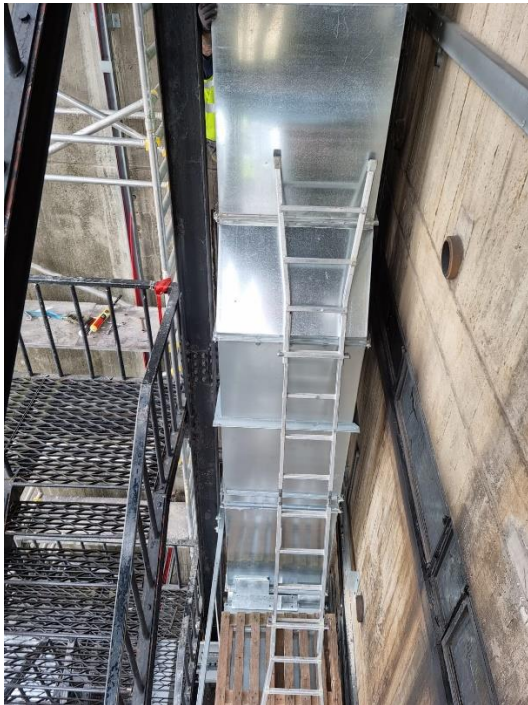
Fire rated ductwork passing through the building
