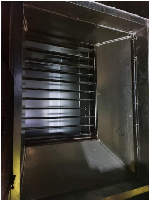
Fire rated dampers to each discharge
