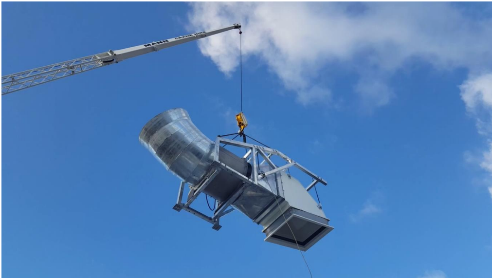
A fan assembly is lowered to the roof of the multi-storey building
